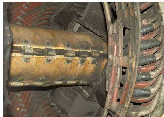
Generator – stator and rotor windings contamination
